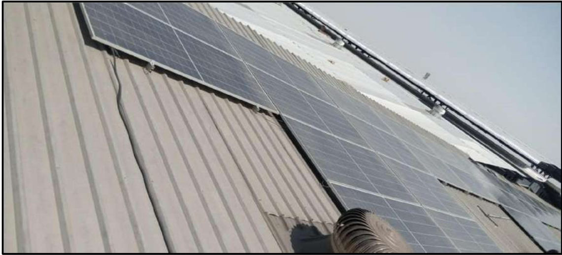
Photographs showing Solar Panels on sheds
